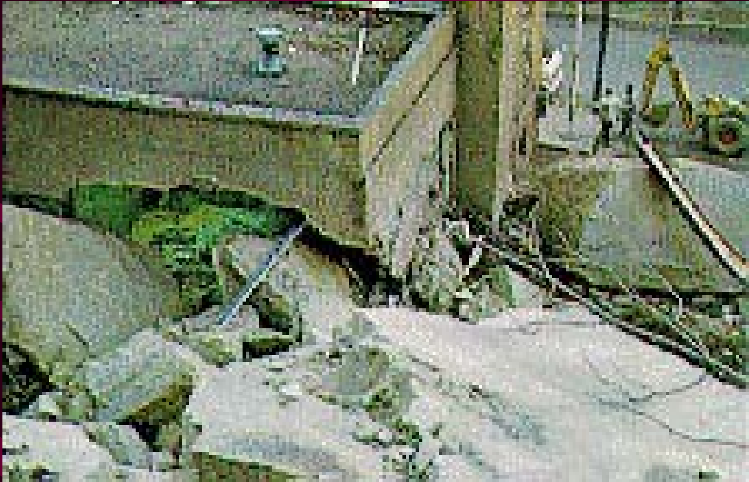
Rockfall at Pomeroy, Ohio
