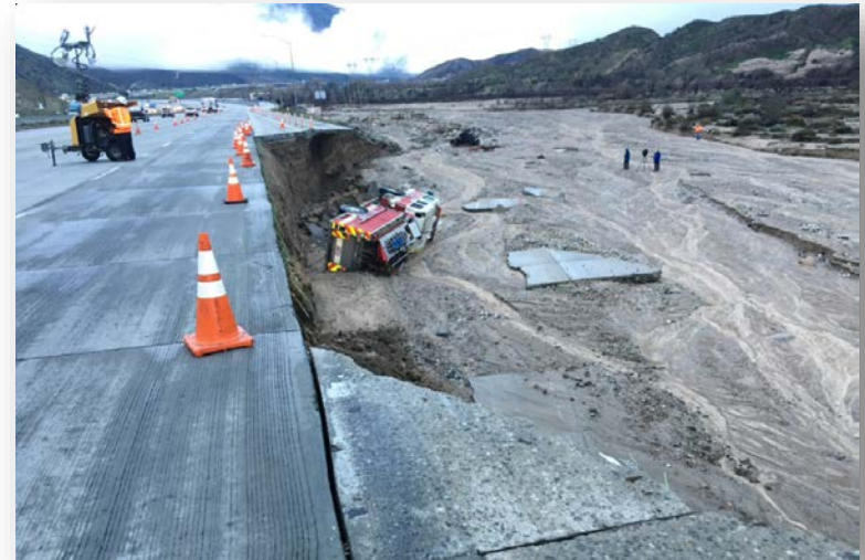
I-15 Cajun Pass Highway Embankment Failure CA (Source: Caltrans District 8)
