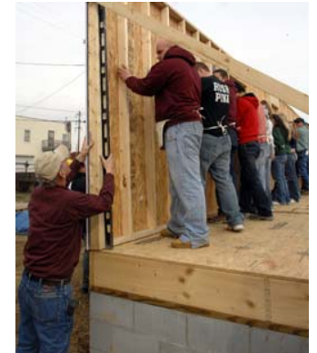
MU Students raise a wall on a Herd Habitat for Humanity house. Photo compliments from MU Communications Dept.
