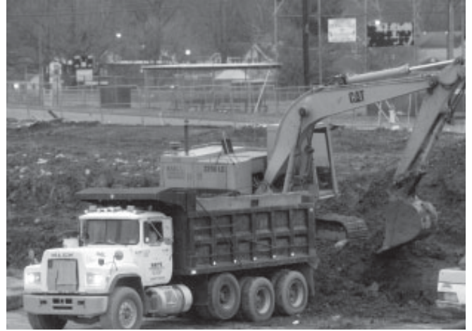
Marshall's old Fairfield Stadium is almost completely history now as the site is prepared for the medical school's Clinical Education and Outreach Center.
