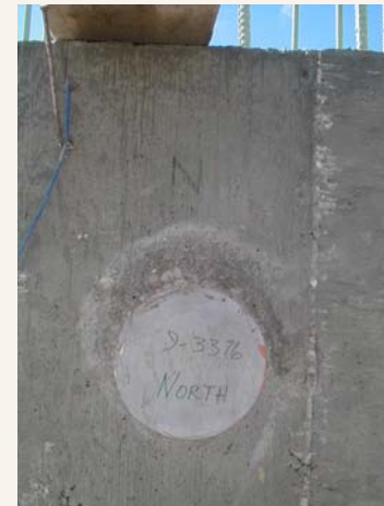
Pressure Cell Cast in Bridge Abutment
