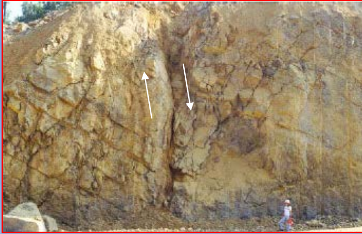
Smart Road Deep Cut Looking North /Northeast. "Possible Fault Zone With Highly Fractured Rock ... Major Instability".
