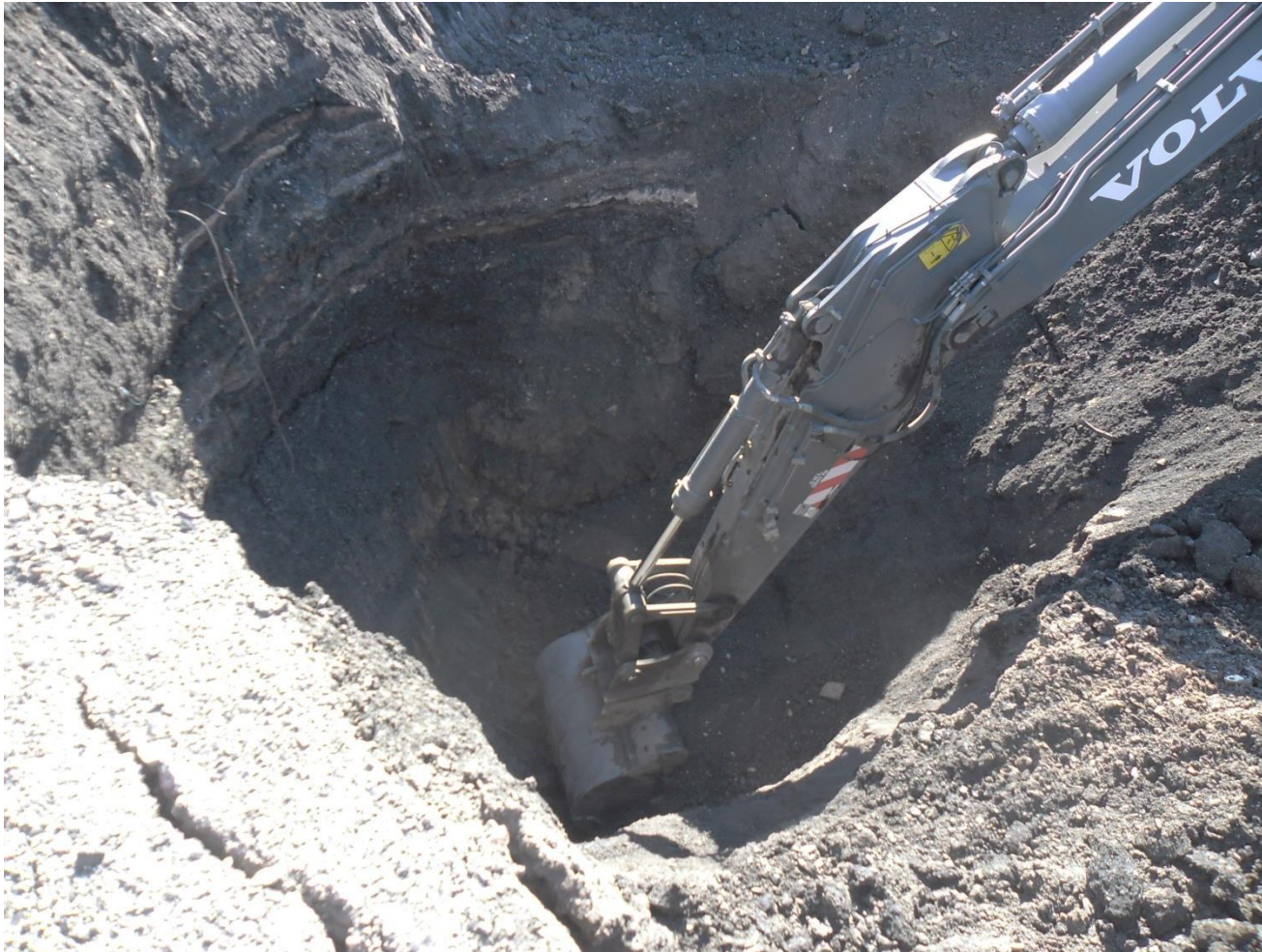
Sinkhole Test Pit
