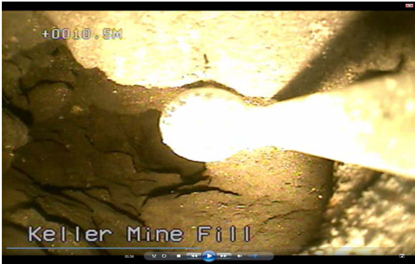
Down looking view showing roof fall in Tunnel 2
