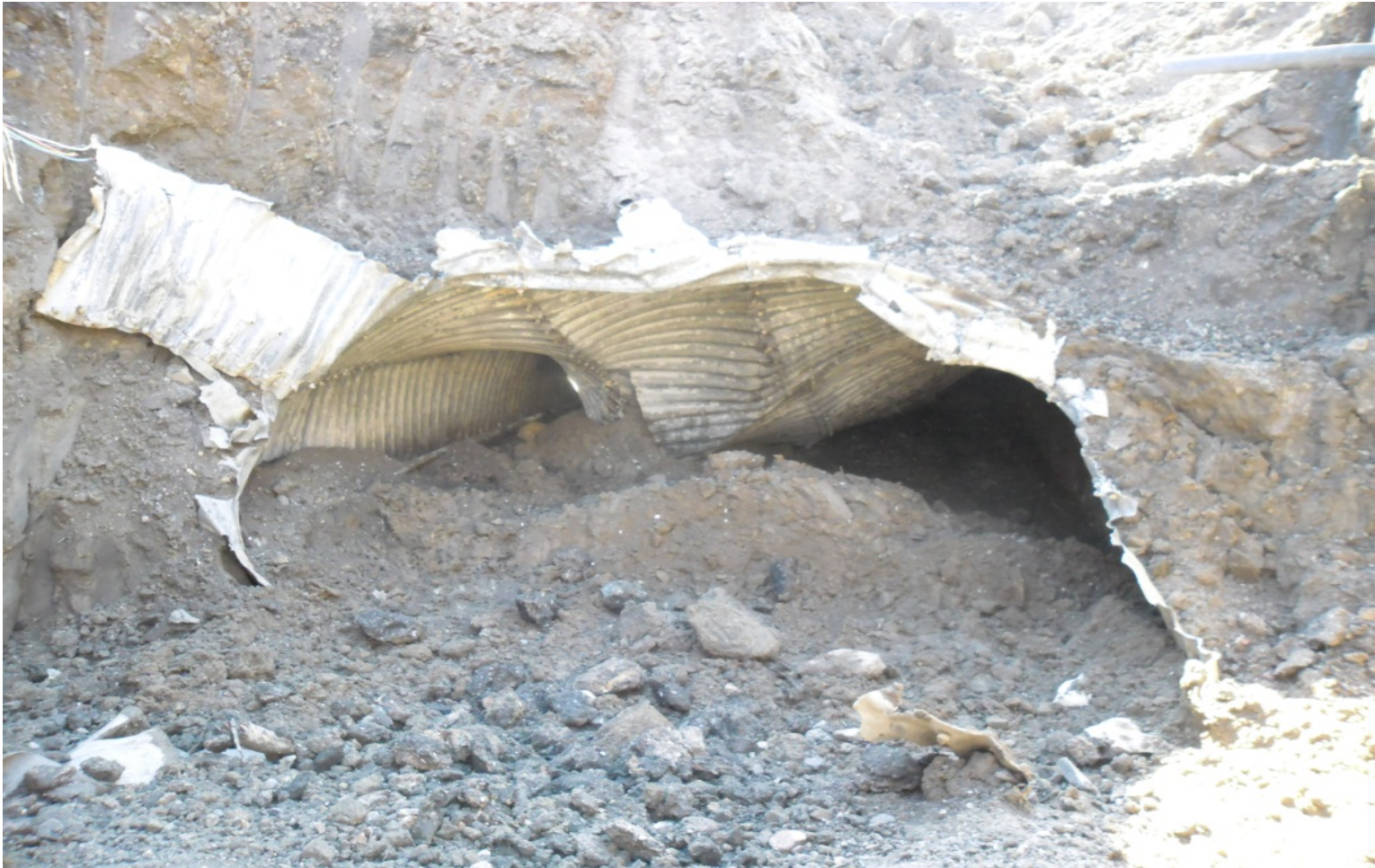
New breach and previous collapse in Old Man & Supply Tunnel (D15) looking downslope
