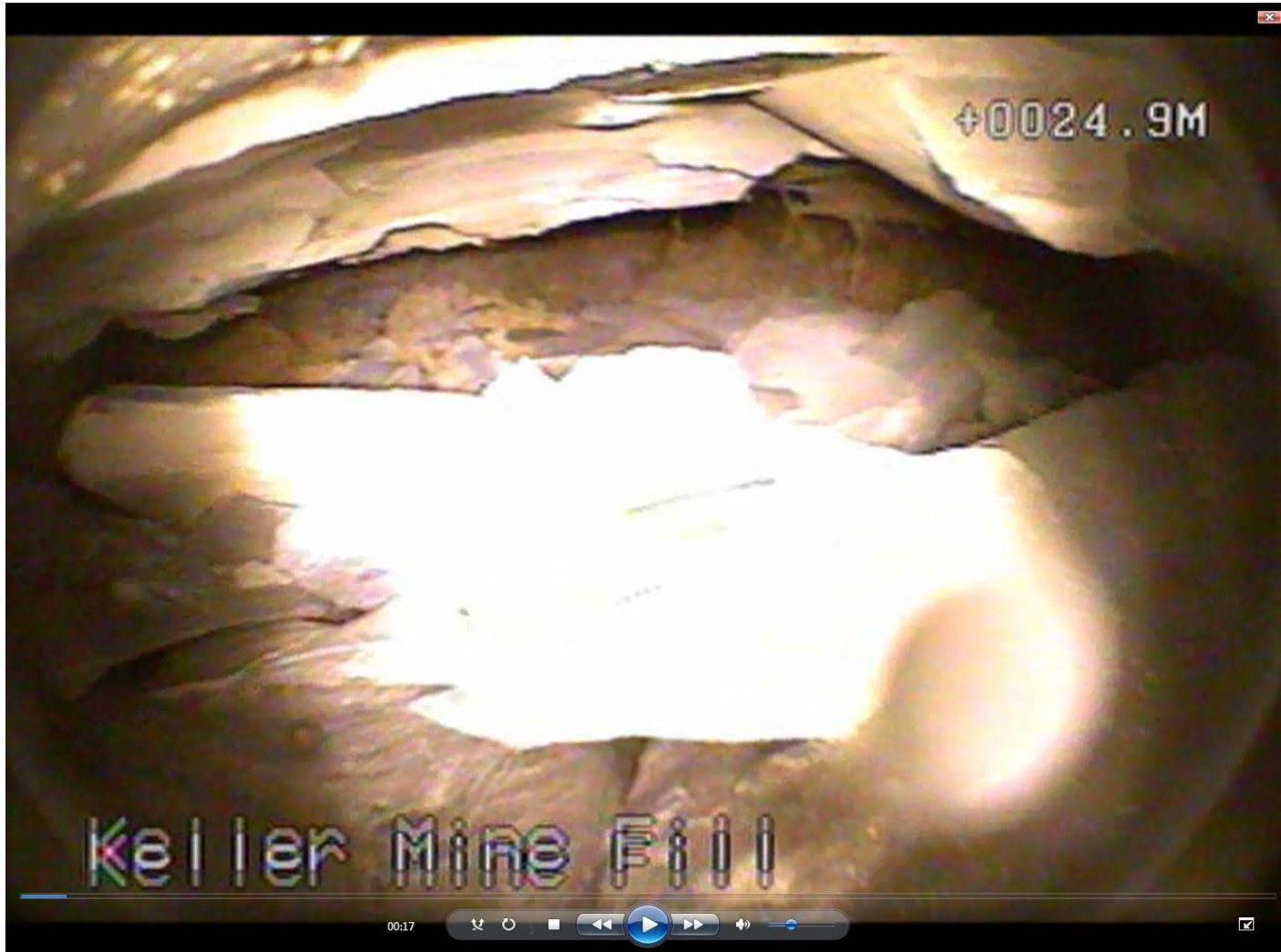
View from borehole camera looking upslope at material from sinkhole in rock tunnel portion of Belt Tunnel
