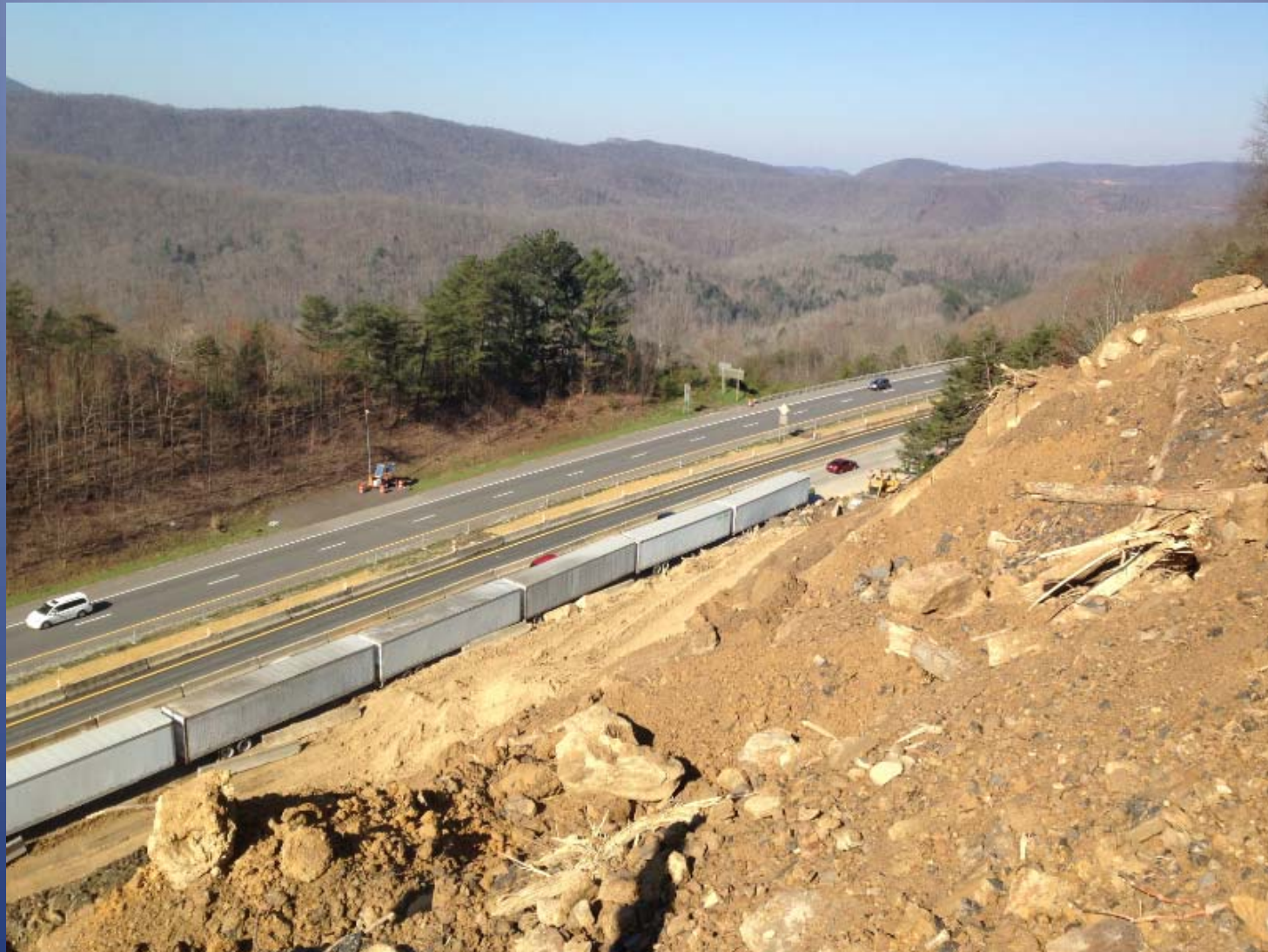
Northbound lanes reopened after construction of temporary lanes in median and removal of the least stable debris 3/26/16
