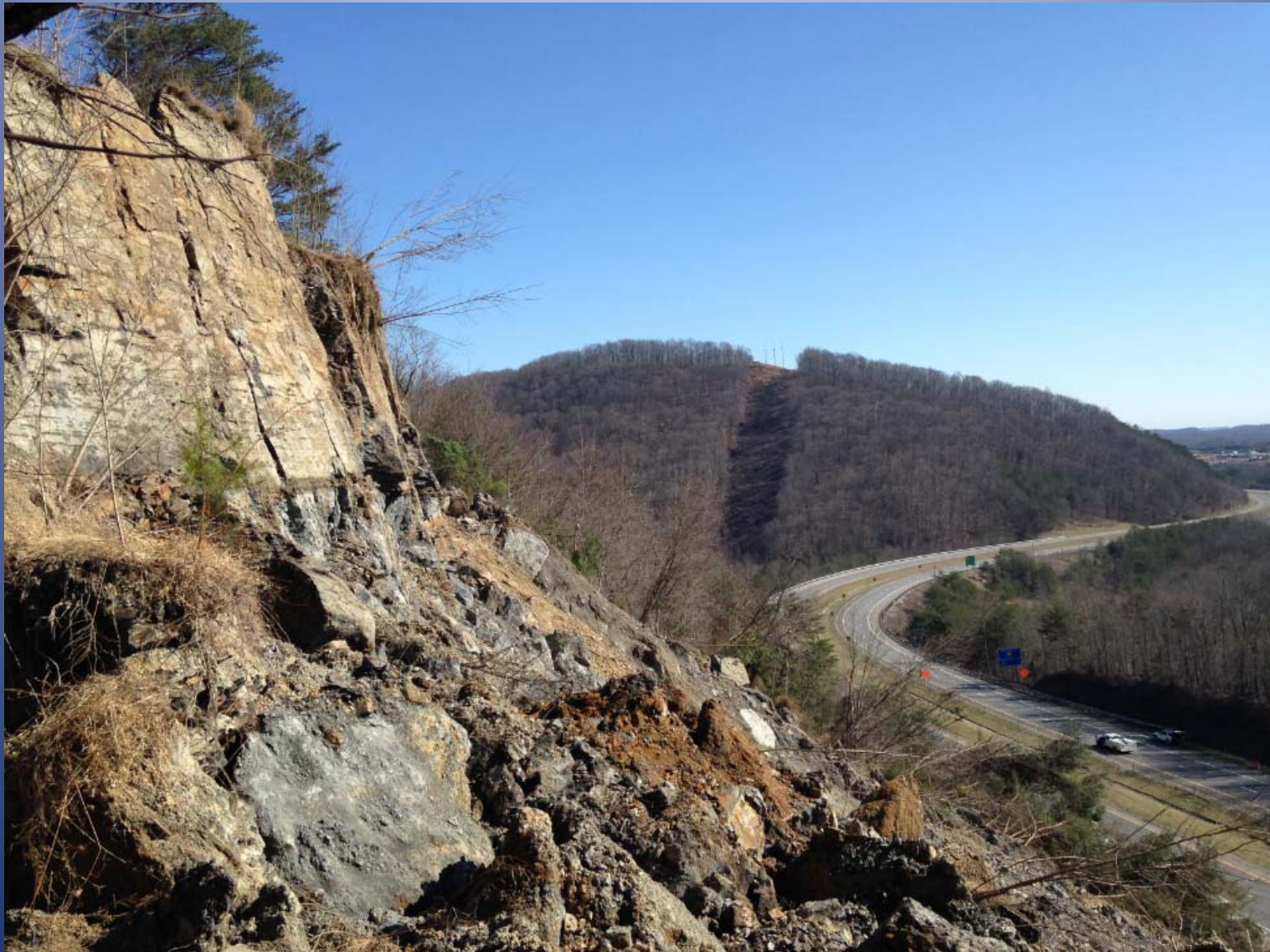
Toe of sliding block looking south
