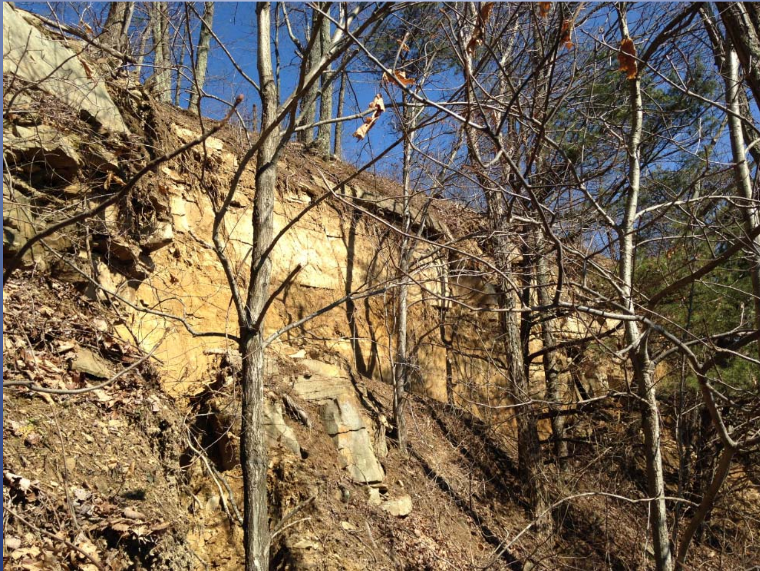
Head scarp/top of release joint/high wall
